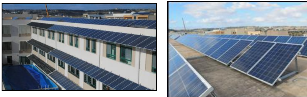
Figure 2: Unglazed pool solar thermal system and PV overhangs on the south courtyard facade (left image) and roof mounted Photovoltaics (right image)
