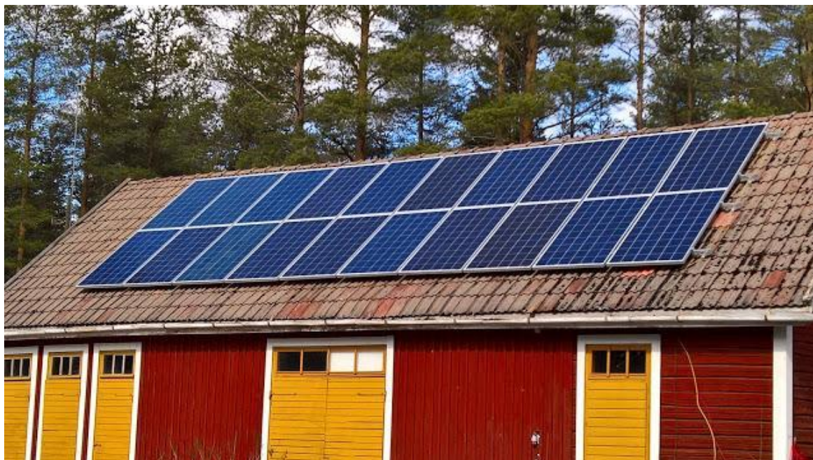
Figure 1. Solar panels on the roof of a building owned by Kätkänjoki village club. Source: Pamaus-karavaanari blog ( http://pamaus-karavaanari.blogspot.fi/p/aurinkosahko-5.html ).
