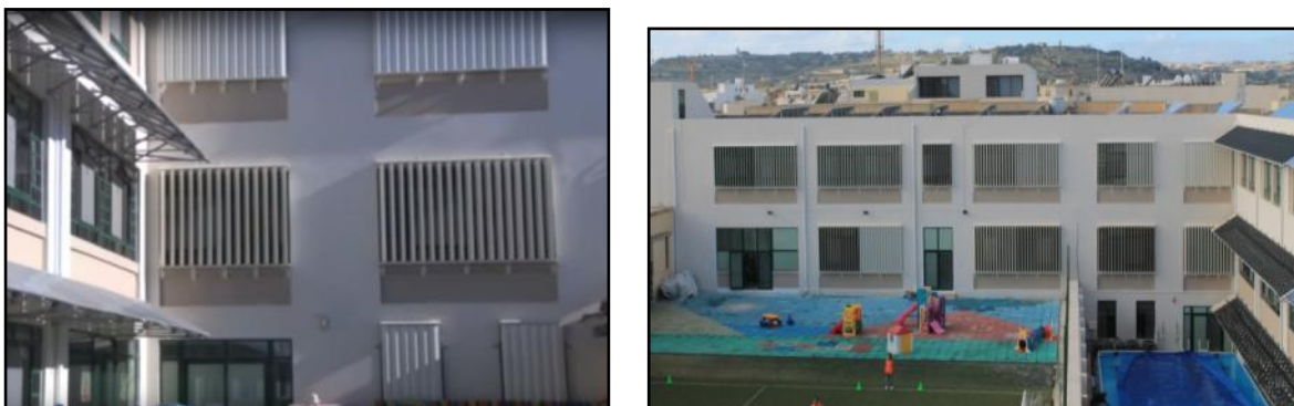
Figure 3: BMS controlled movable external vertical louvers on the East and west facades
